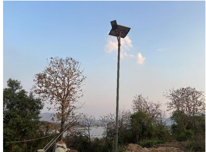
Figure 21: Street solar lights
