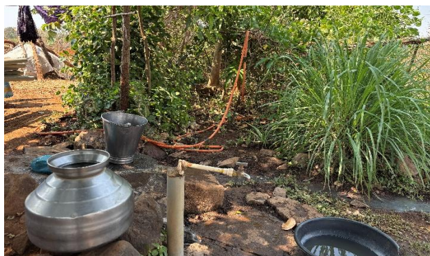
Figure 9: Water supply tap in Somaj village
